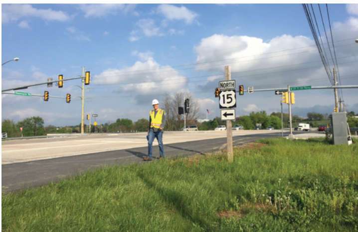
Steve at the installation of the first flashing yellow arrow in Pennsylvania.
